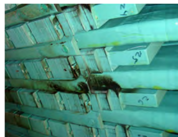
Fig 6: Photograph of a 150 MVA hydrogen-cooled turbine generator that had extensive greasing at the slot exits due to loose bars in the slot. The side packing was also abraded. The associated PD data is shown in Fig. 5.
