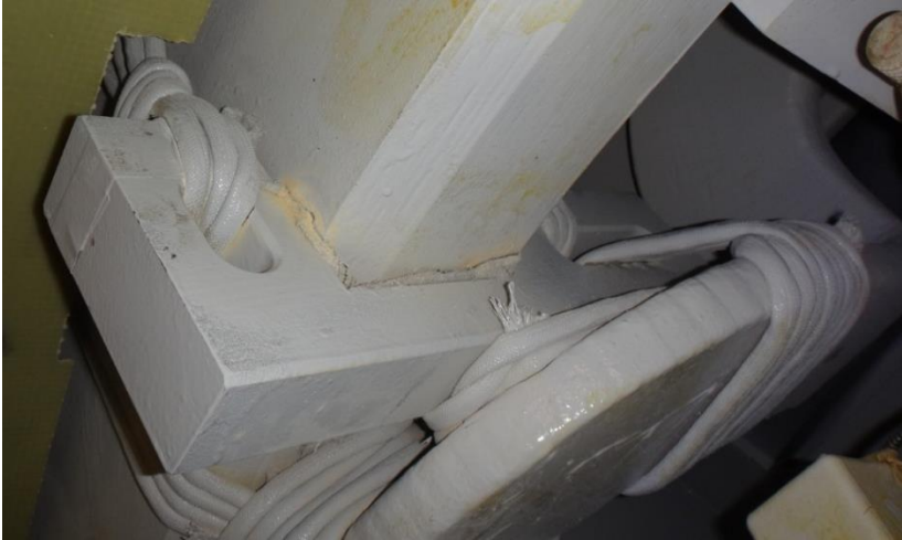
Figure 4 – Loose blocking near 11:00 Jumper Connection
