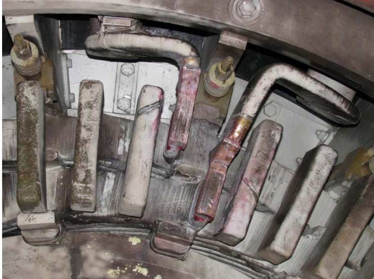
Other as found blocking & phase lead connection exciter end
