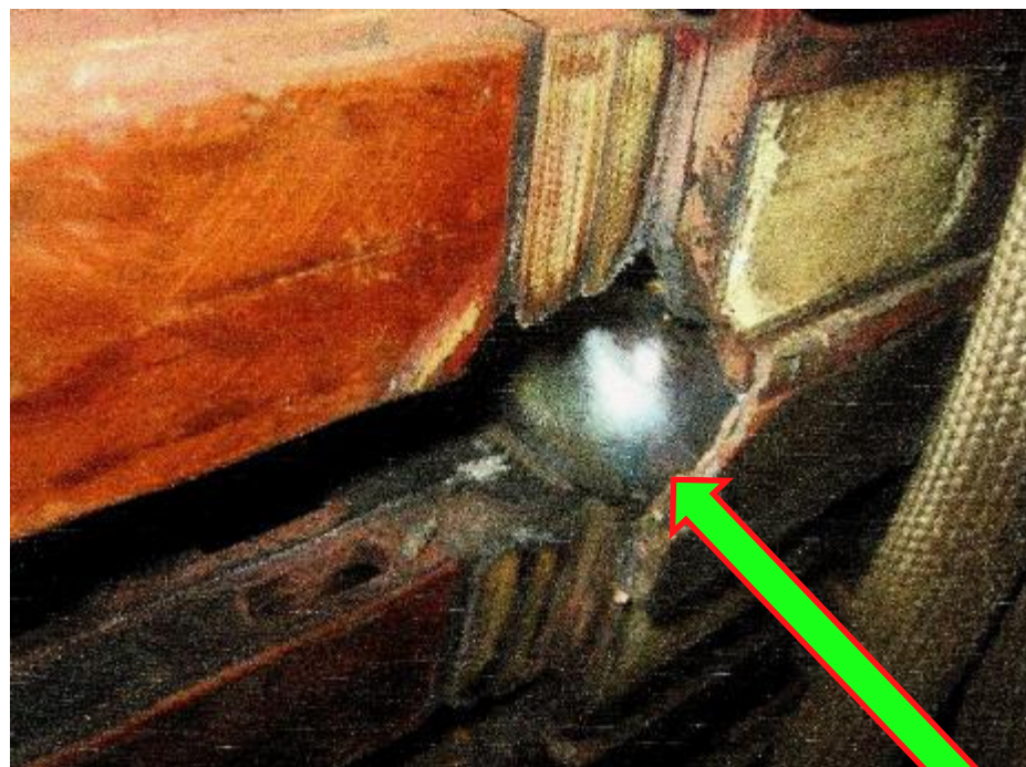
Rotor coil and forging arc fault damage (exciter end)
