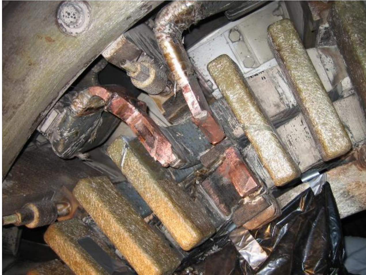
11 o'clock position where initial arc flash over occurred
