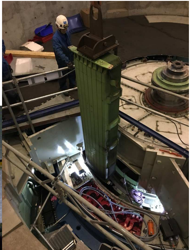
Faulty pole being removed
