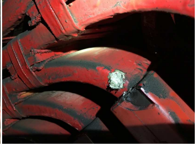
Impact on stator winding
