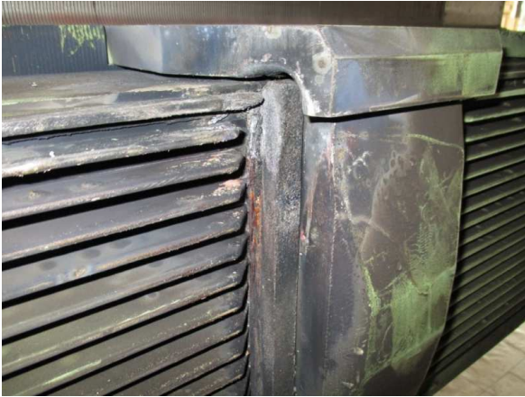
Pole 1 with arcing evidence between winding and body
