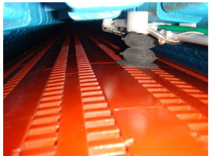
Fig. 10. TF probe installation with rotor in situ .
