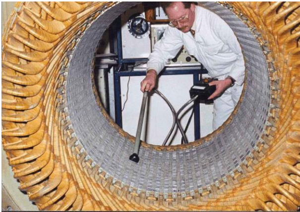
Fig. 4: Example of a corona probe test on a stator winding
