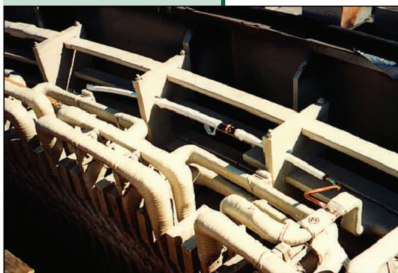
Figure 1: A photograph of an 80 pF "cable-type" coupler (in the process of being installed) that was widely used in the 1980s to detect the PD on hydrogenerators.
