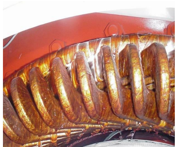
Figure 7: The white powder (fretting) on this motor stator endwinding is caused by relative movement between the coils and the endwinding support ring.
