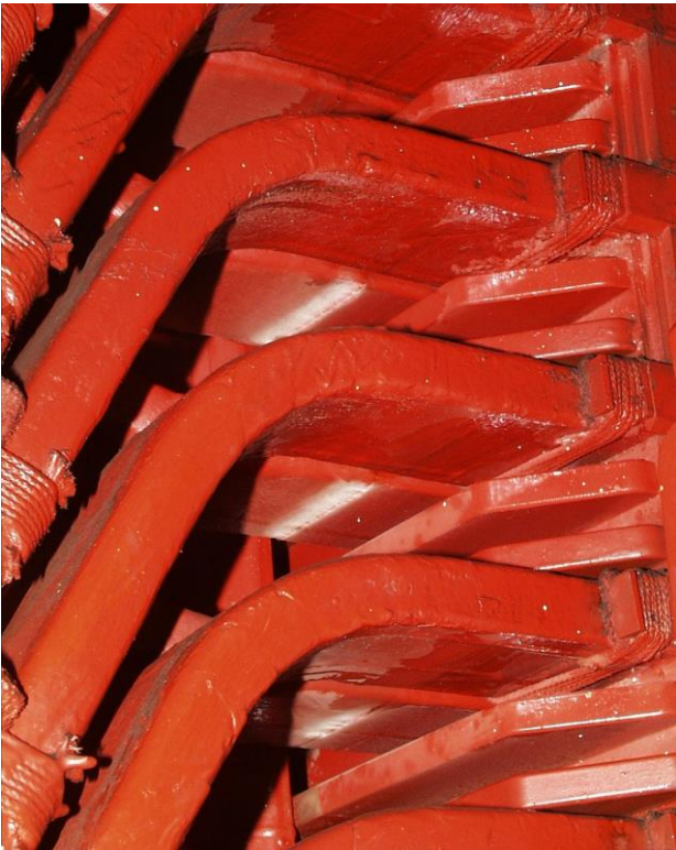
Figure 2: Semicon and grading coating overlap deterioration (white powder) due to poorly applied or inadequate coatings
