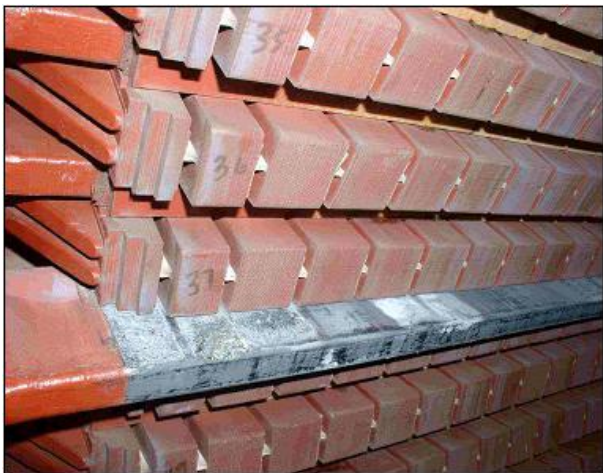
Figure 6: Bar abrasion due to loose windings in the slot of a turbo generator that did not have sufficient sidepacking or a radial follow-up wedging system. The bar is in the process of being removed after failure.
