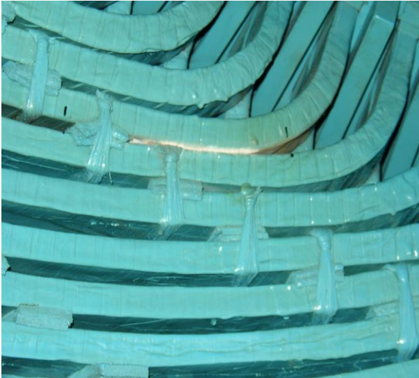
Figure 5: PD occurring between high voltage coils in two different phases, where the spacing is insufficient to prevent the PD. Note that the spacing between adjacent coils is irregular, as a result of poor manufacturing processes.
