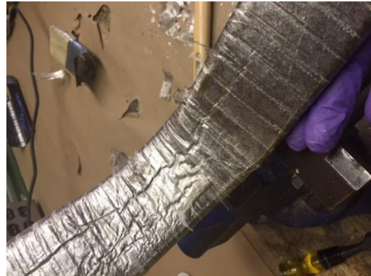
Fig 10- Excess wrinkles resulting from lack of tape tension
