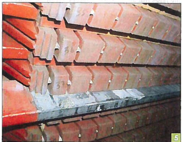
Coil abrasion due to loose windings in the slot of a turbo generator. The coil is in the process of being removed from the core.
