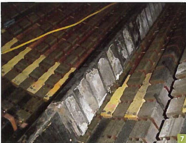
A neutral-end stator bar damaged by vibration sparking. The bar is in the process of being removed from the slot.
