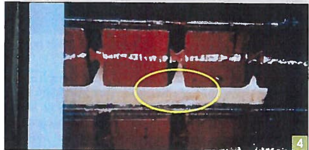
Destruction of the coil semicon coating in the stator slot due to PD and ozone.
