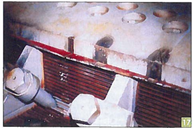
Top pole washer failure from mechanical forces.
