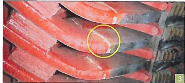
Semicon and grading coating overlap deterioration.
