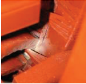
Figure 1: Winding bar insulation abrasion at support ring
