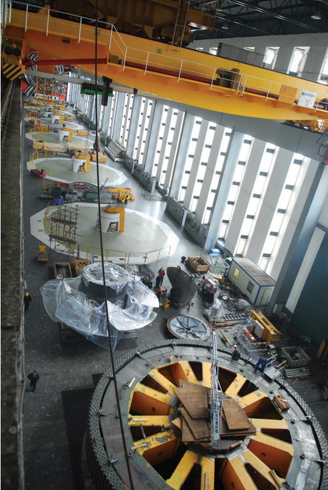
Pict.No 3 – The hydropower units - Machine hall.
