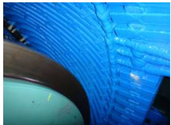
Fig. 2 Dusting on stator endwinding near the 5 o'clock position top connection
