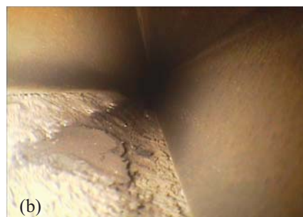
Fig. 5a. and b. Borescope vibration sparking damage to stator bar insulation.
