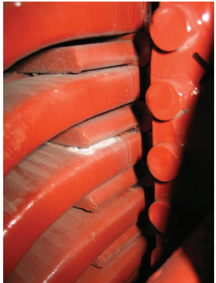
Figure 3. Powder deposit attributable to partial discharge (PD) occurring between a motor stator core pressure finger and a coil.
