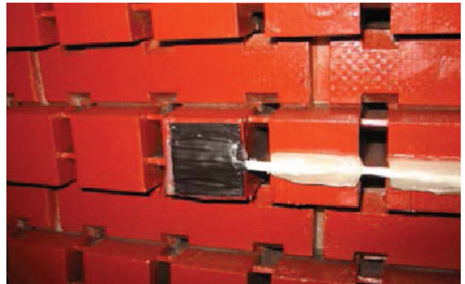
Fig. 2 Commercial airgap search coil installed on stator tooth surface for detecting short circuits in field winding of synchronous machine [17]
