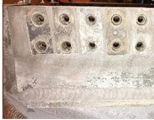
Photo 3. Arcing damage to bus connection surfaces.
