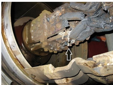
Photo 4. Failing flexible connection joint.
