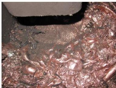
Photo 6. Many pounds of melted copper from this connection failure.
