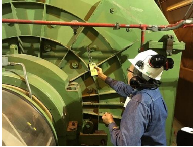
Photo 15. Checking the end of a generator for radiated EMI.
