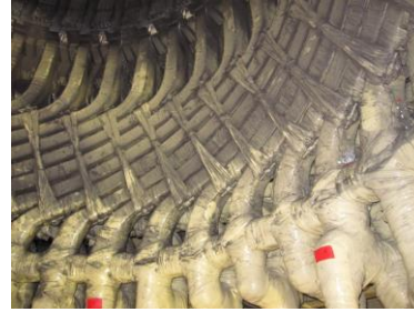
Photo 7. Resulting contamination to stator winding.
