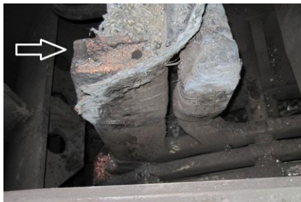
Photo 5. Remains of failed connection.
