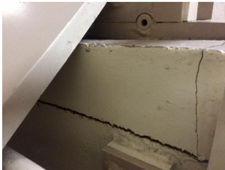
Figure 11 – Cracks in bearing to foundation supports on other unit in the same plant
