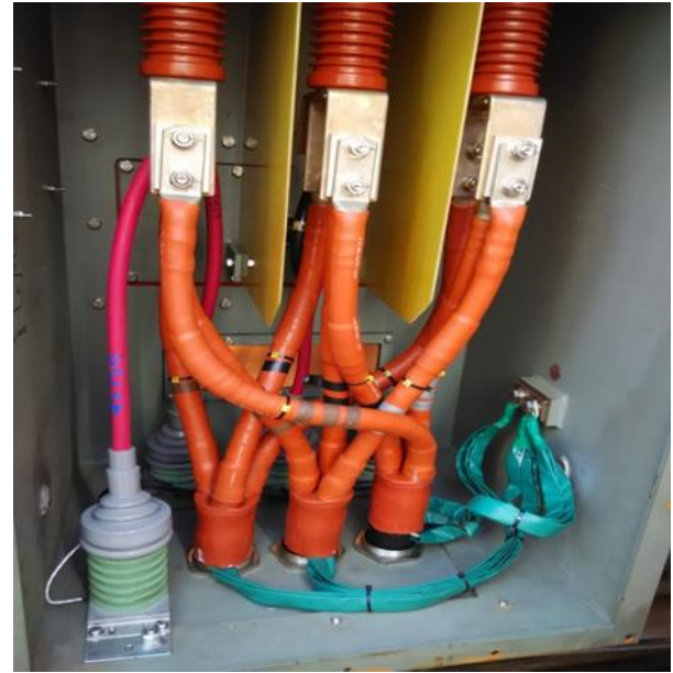
Figure 6 Installation of 3 PD sensors and a voltage divider in the terminal box of an IFM.
