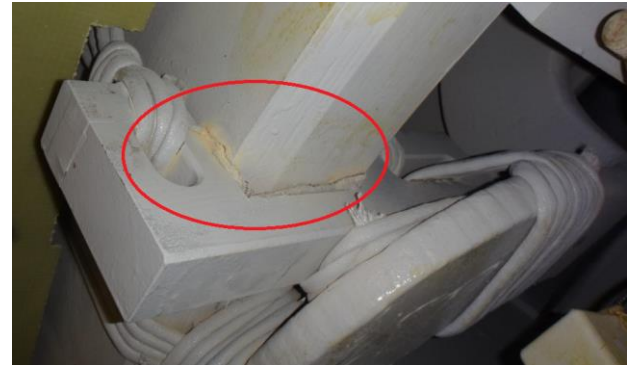
Fig. 7 – Loose blocking near 11:00 Jumper Connection [8]
