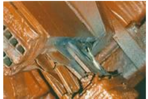
Figure 1 – Failed phase connection [1]
