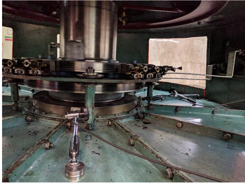
below slip-rings, above thrust collar
