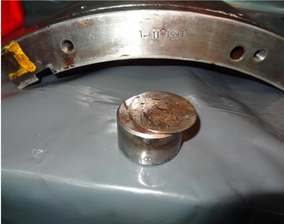
Vibration caused damaged pads (used to set bearing clearance) on LGB
