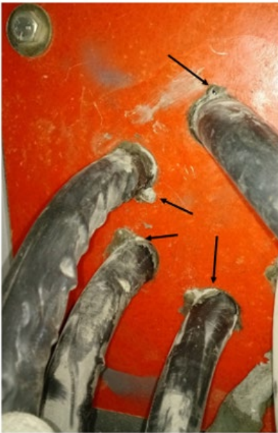
Severe Discharging at Lead Support
