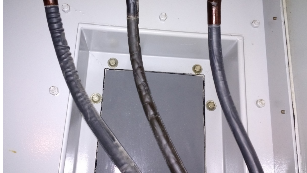
Grossly Overheated Lead Insulation
