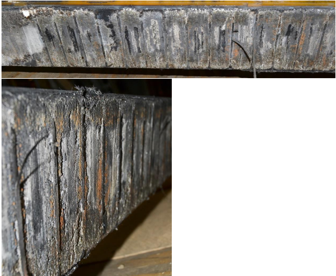
Picture 1. Failed stator winding bar of Case 1. The crater-like appearance is clear sign of sparking, caused by slot discharges or more likely vibration sparking.
