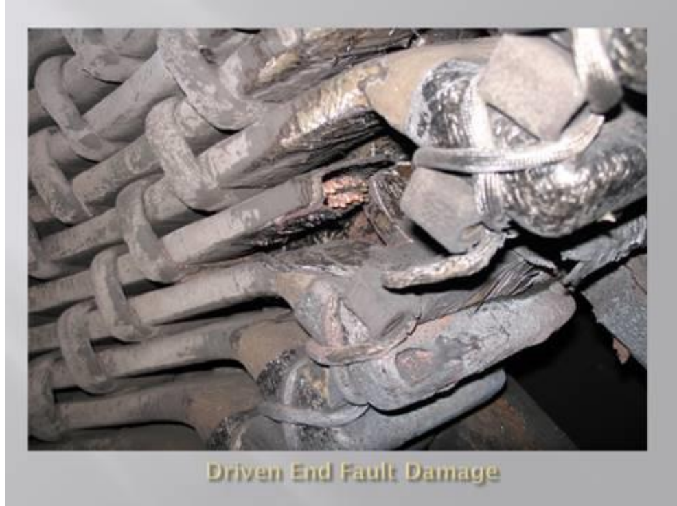
Failure of stator coil end turn
