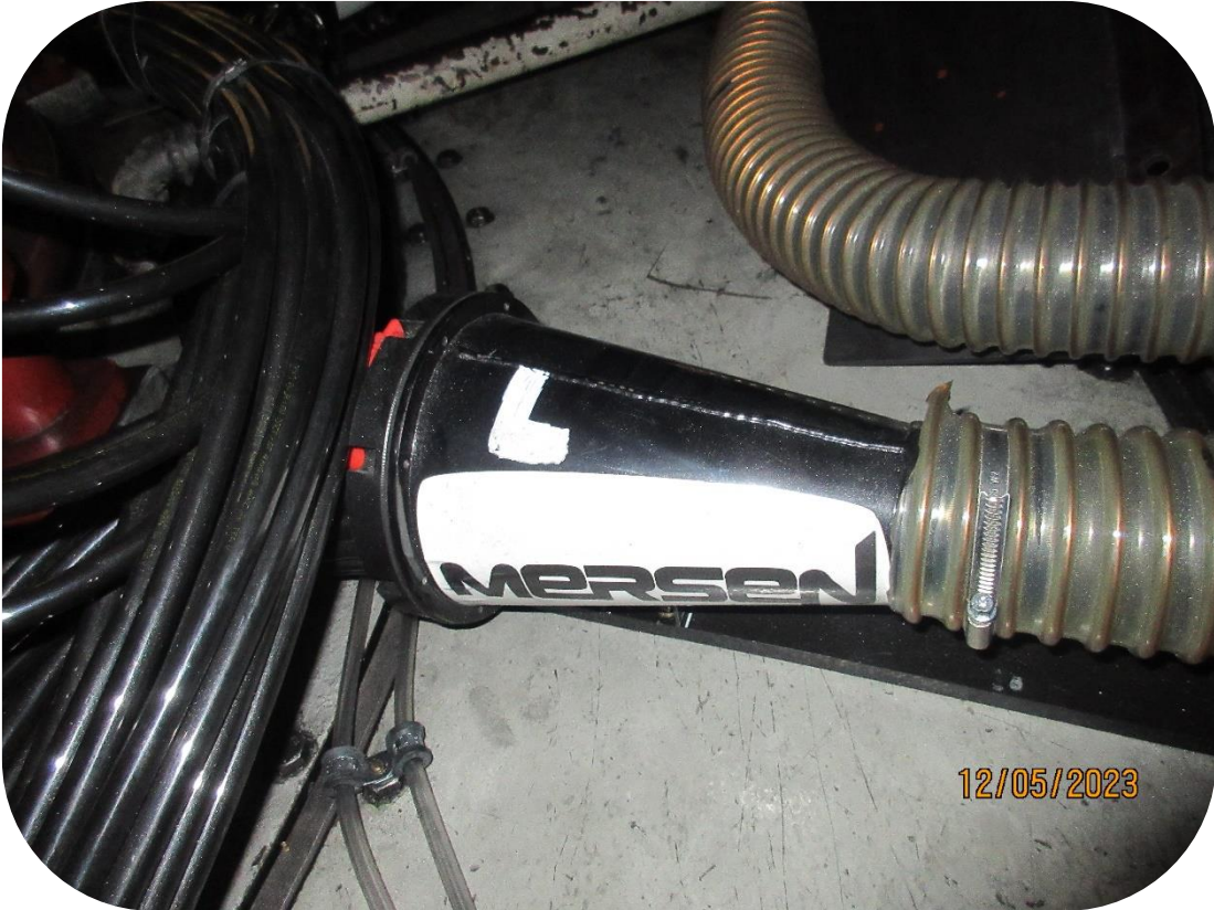
Vacuum Piping Manifold
