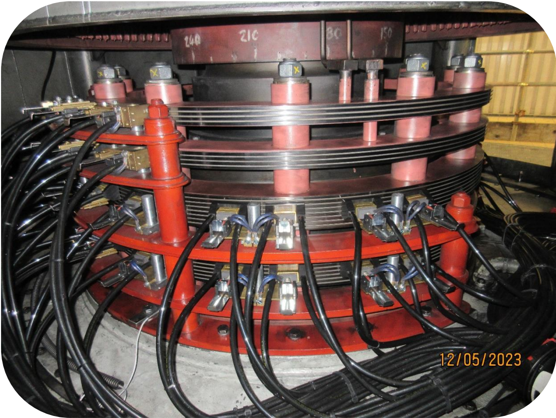
ESB Turlough Hill Installation
