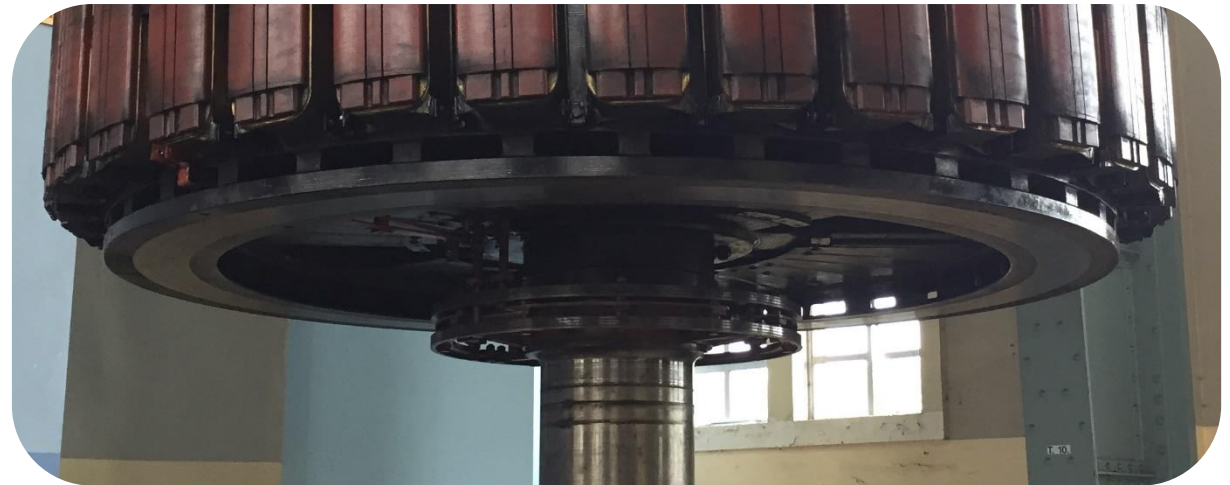
Slip rings located beneath generator rotor. Rotor cooling fans located at top and bottom.
