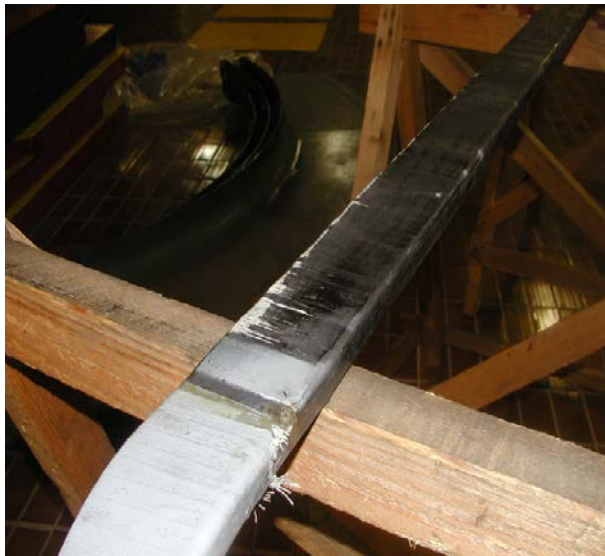
PD on interface semi-conducting and gradient coating (coating deterioration)
