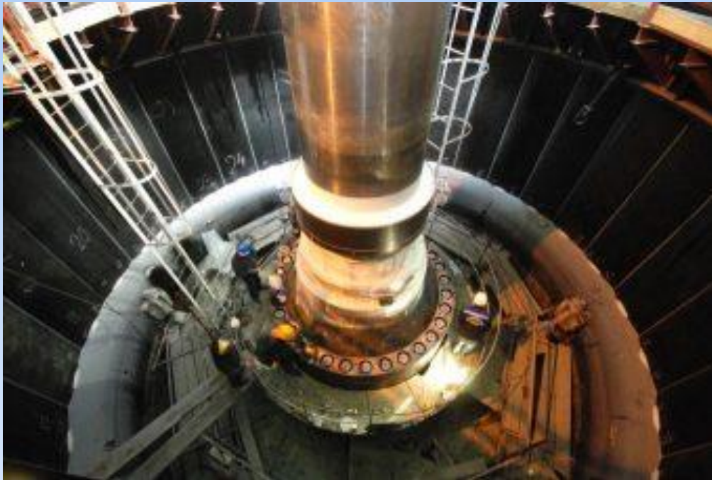
Turbine shaft: 10 m long, diameter 1, 6 m and 90 tons weight, connects the runner blades and generator rotor.
