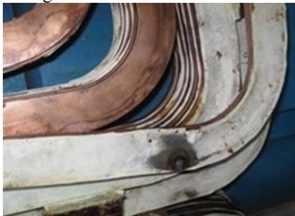
Fig.3 Failure spot around the corner
