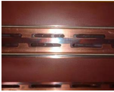
Fig.2 Failure spot close to the vents
