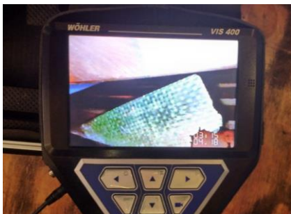
Fig.4 Displacement of the inter-turn insulation
