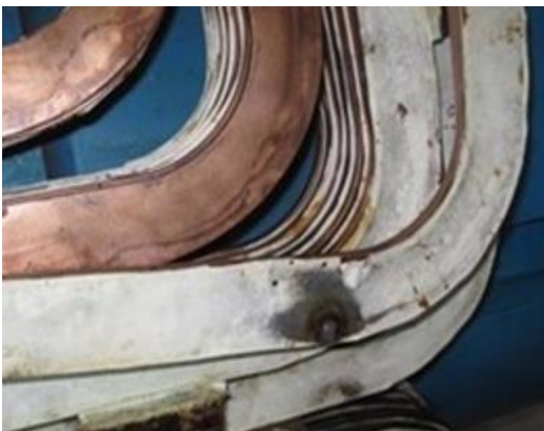
Failure spot around the corner
