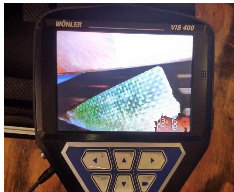
Displacement of the inter-turn insulation
