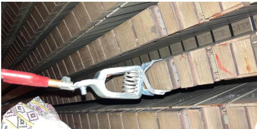
Picture 8. The core is connected to the DC plus.
