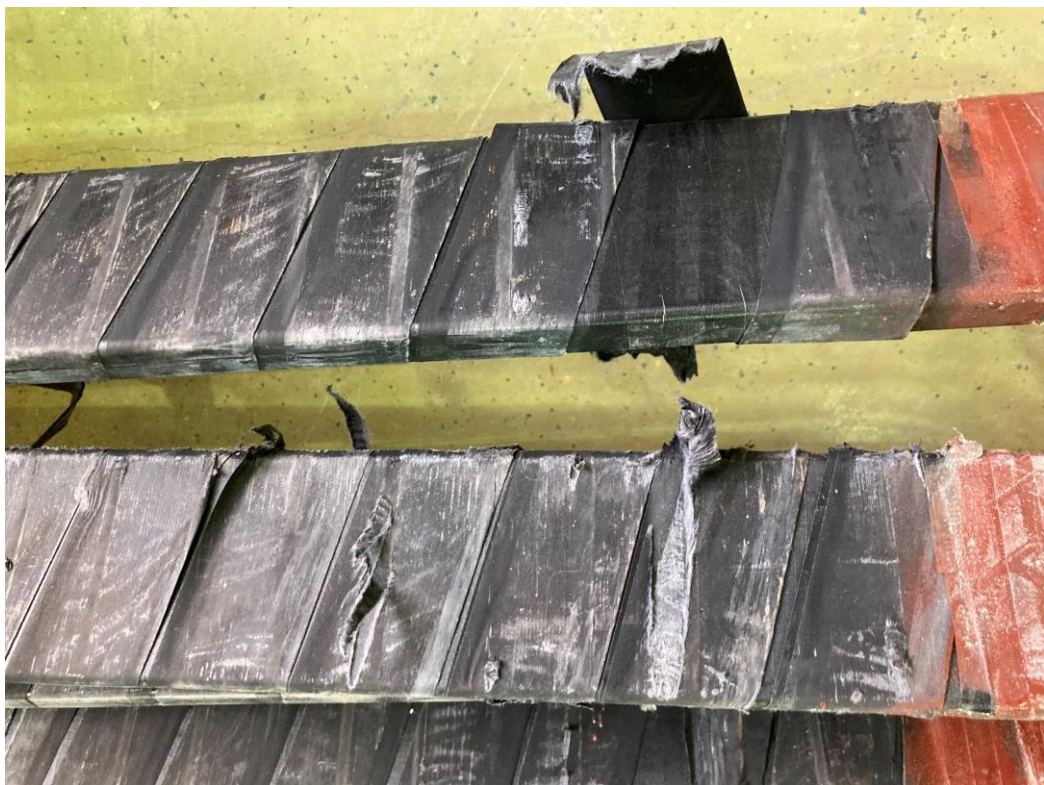
Picture 2. Round packing type of fitting on the removed stator winding bars.
