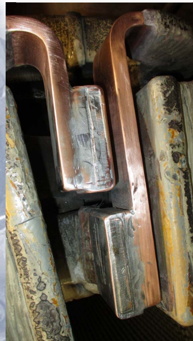
Undamaged Phase Connections
