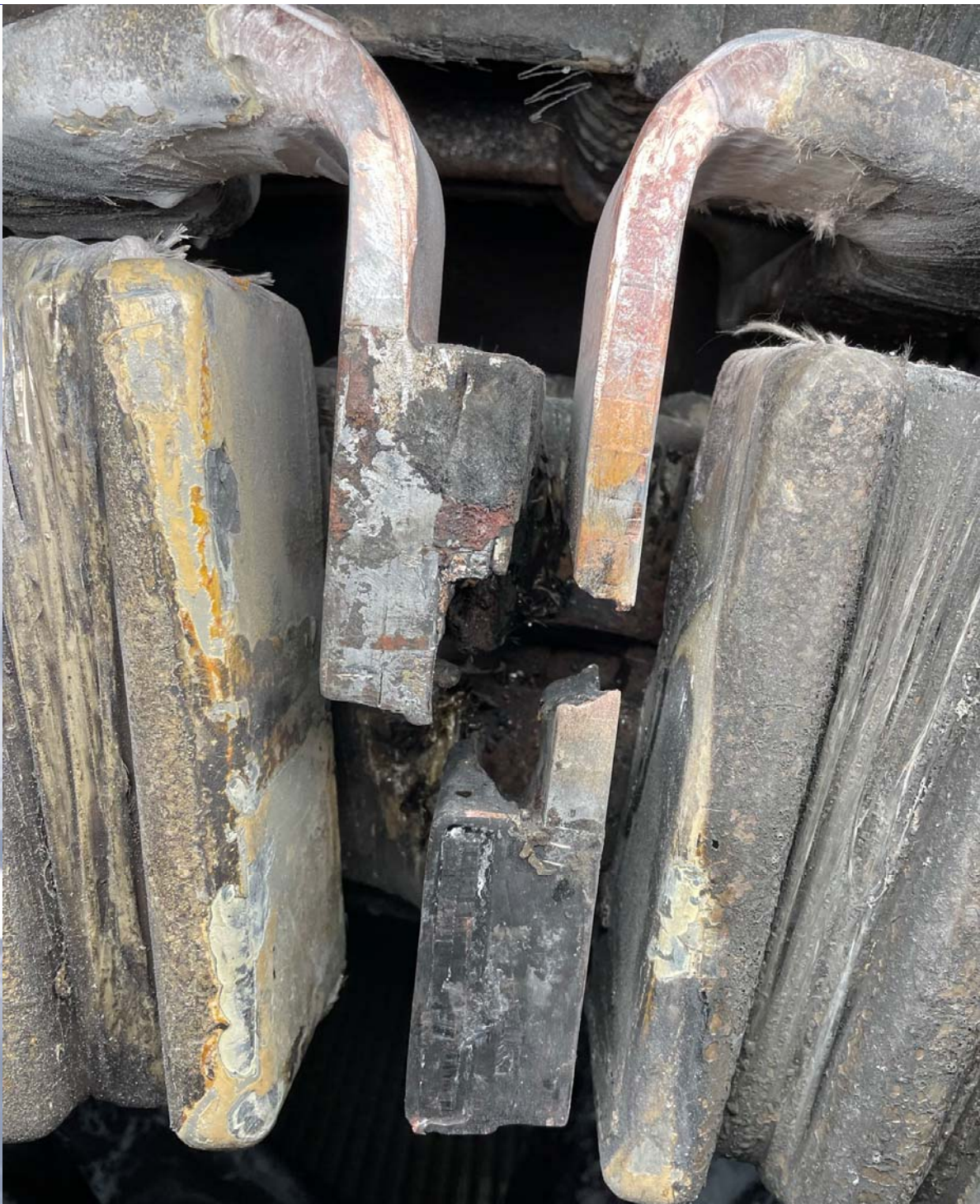
Damaged Phase Connections
