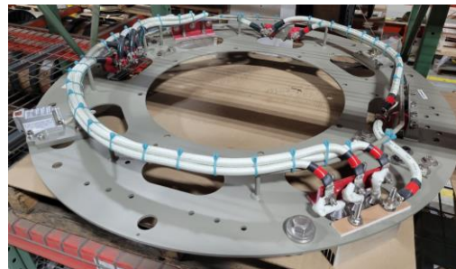
Diode wheel rectifies AC to DC and supplies DC power to the main rotor field
