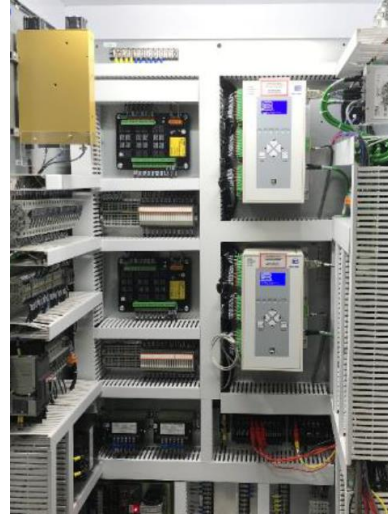
The AVR controls excitation current and supplies DC power to the exciter stator
