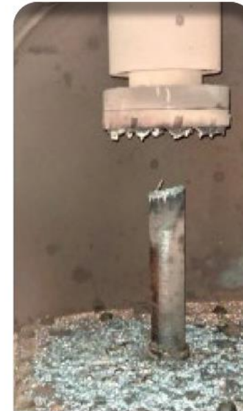
Figure 1. Photo of main lead failure. EPRI TGUG Generator Workshop Presentation, "Wise County ST Generator Main Lead Failure, Stephen M. Bates, August 15, 2022. [4]
