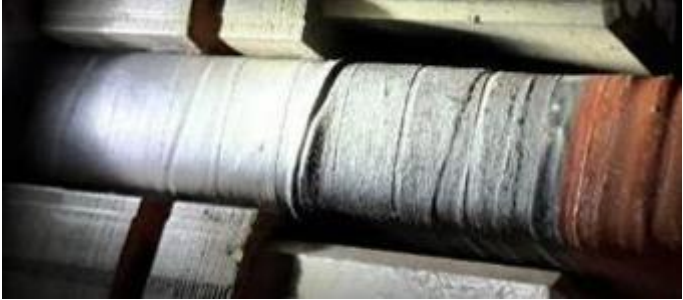
Photo of GVPI bar “ridge” concern in 2022 EPRI Generator Workshop presentation by Duke Energy
