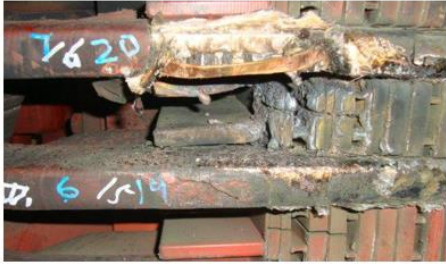
Failure & Rewind of a GVPI Generator – EPRI Australia Workshop, 2015 by W. Moore
