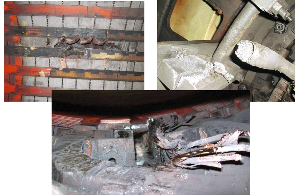
Ground fault failures shown in 3002024098.
