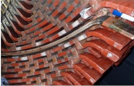
GVPI Stator Bar Failure 2022 TGUG by D. Fischli, Duke Energy
