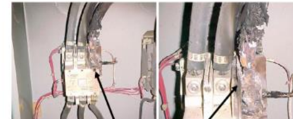
Evidence of severe arcing
