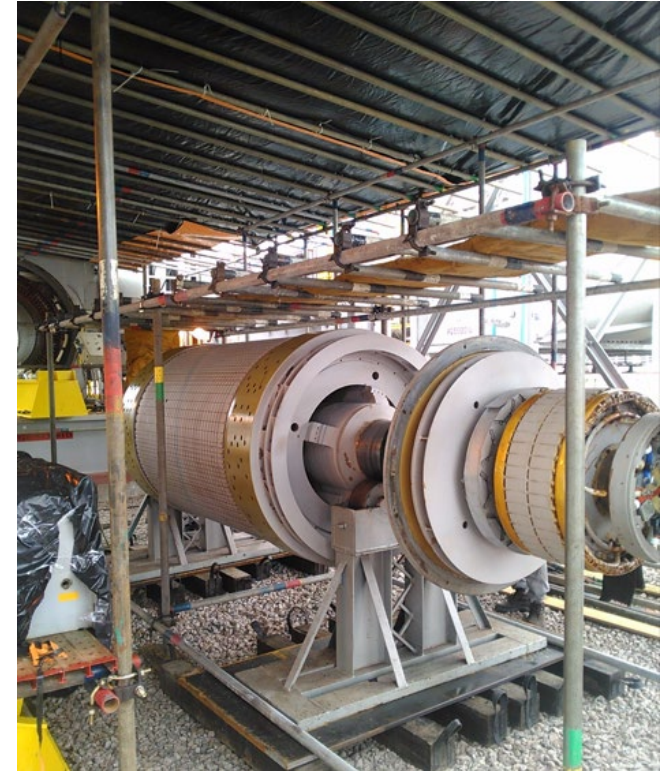
Structure to accommodate and cover the rotor
